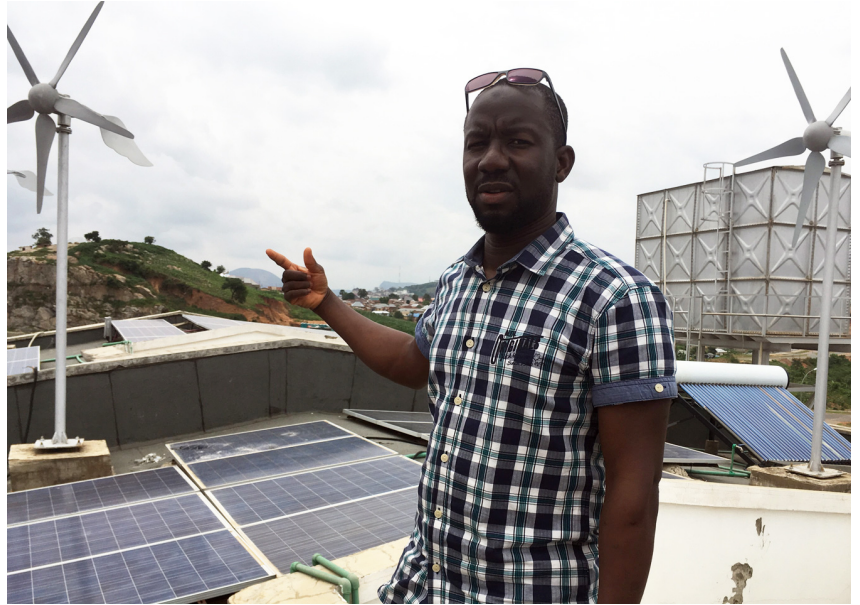
Abdrahamane Traoré stands near the wind/solar/battery microgrid he helped optimize at an apartment complex in Nigeria. The project was done in collaboration with a energy company and was part of Traoré’s dissertation for his Ph.D. in Systems Engineering.
