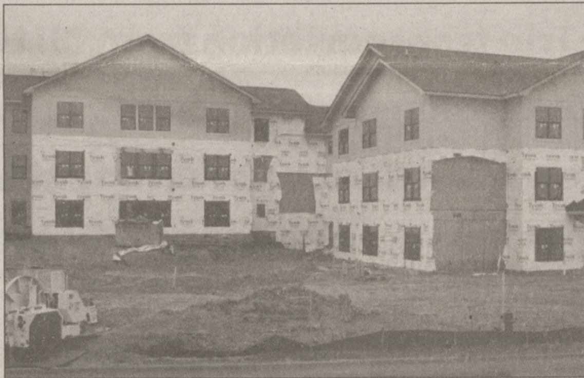
MOVIN' ON UP: The new student apartments are well under construction and will open in the fall. If the Board approves the revised contract, Comcast will provide cable services to the apartments.
