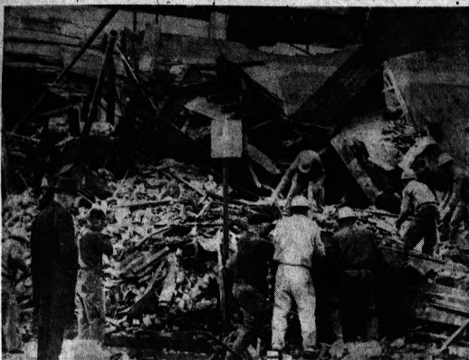
TEN HURT — Workmen probe ruins of a three-story Boston building that exploded yesterday injuring at least 10 persons. The structure was being demolished when a gas leak apparently caused the blast.
