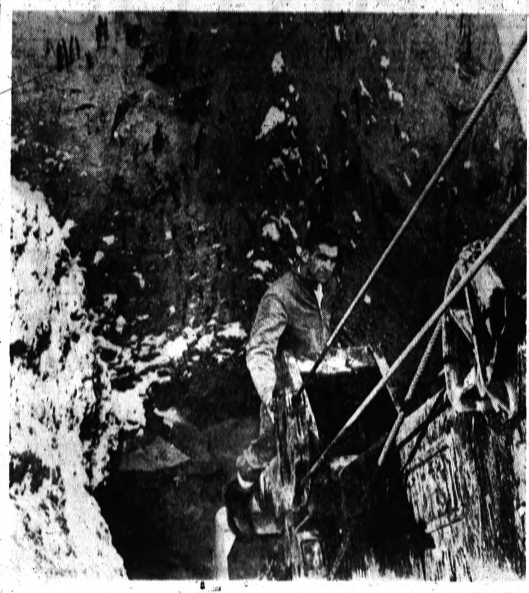
LEAKY PIPE: County Courthouse maintenance men have been working to repair a broken water main into the building since last Wednesday. Andy Vagasceno, 4265 Meyers, Waterford Township, is seen standing near the bottom of an 18-foot hole where the break finally was located. Workers expected to have the 4-inch water main repaired by tomorrow. Meanwhile, water is being supplied into the building by a temporary hookup.
