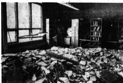
SCHOOL IS INTERRUPTED — Someone has a mess to clean up before school can resume in Seward, Alaska. This was left behind after Friday's earthquake. The rubble on the floor is mostly the result of the ceiling tiles being shaken loose by strong tremors.
