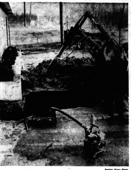
DEATH SCENE — One man was killed and two others hospitalized when gas in this well hole at Morey's Golf and Country Club, 2280 Union Lake, Commerce Township, overcame them at about 6:30 a.m. today. The men had poured acid in the well to blow the point and were uncapping it when gas escaped.
