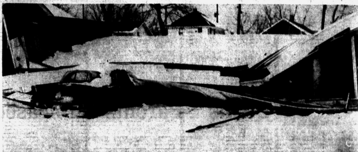
SNOW COLLAPSES GARAGE ROOF — The heavy load of ice and snow piled by winter on this garage roof simply became too much for the frame structure to hold up. Used for storage by Hol-
