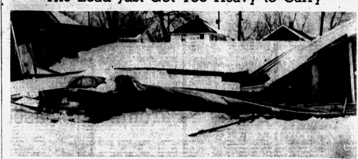
SNOW COLLAPSES GARAGE ROOF — The heavy load of ice and snow piled up on this garage roof simply became too much for the frame structure to hold up. Used for storage by Holterback Auto Parts, the building, located at 273 Baldwin Ave., yesterday afternoon collapsed. This car and another were damaged, but no one was reported injured.
