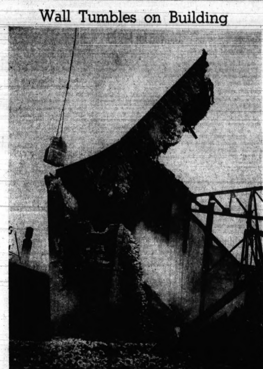
AFTERMATH OF FIRE —Demolition crews yesterday were battering down masonry brick walls of the fire-gutted Oakland Theater on S. Saginaw Street when tons of brick tumbled through the roof of the adjacent Yankee Clothing Store warehouse. The south wall was being hammered with a huge crane swung weight when the lower half buckled outward as shown here. An estimate of damage to the warehouse and stock inside hasn't been determined yet. The Capital Wrecking Co. of Grand Rapids had been contracted by W. S. Butterfield Theaters Inc., owners of the Oakland Theater, to tear down the ruins.
