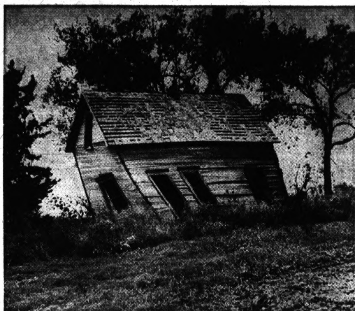
THE WIND BLEW THAT-A-WAY—This old house, sitting on a knoll near Goodrich, Kan., was once a waystation for early-day settlers crossing Kansas. Typical of the many frame dwellings that once dotted the prairie, the house is succumbing to time and the elements.
