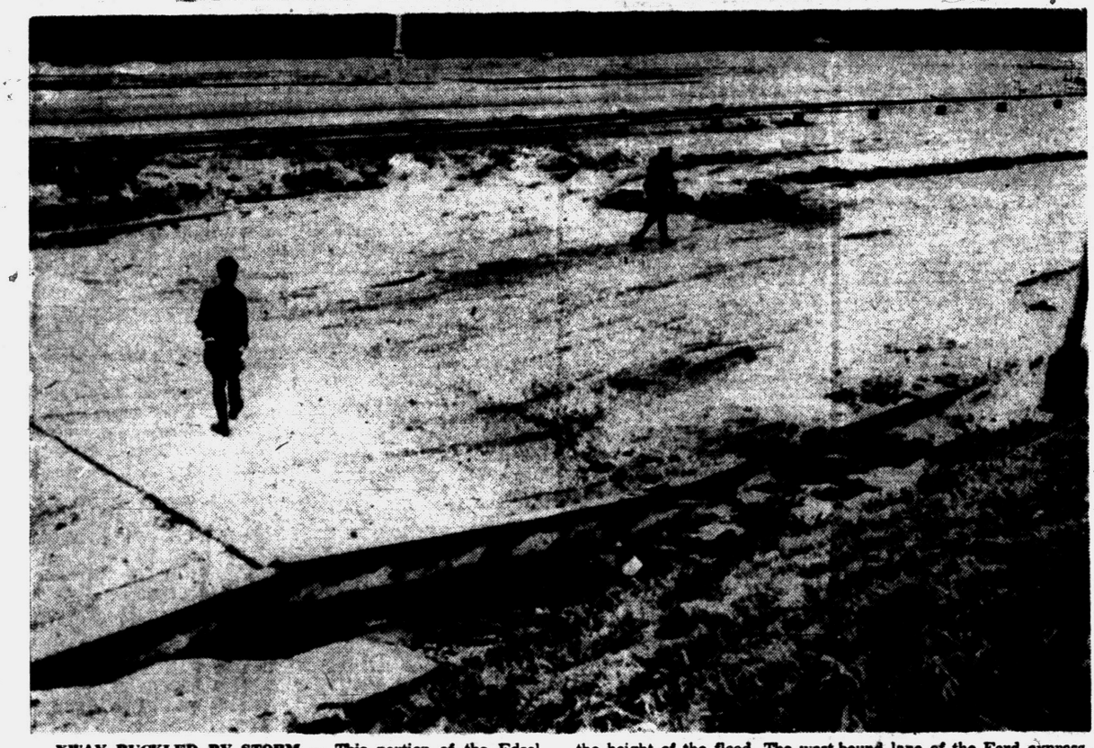
HWAY BUCKLED BY STORM —This portion of the Edsel Ford Expressway was left a twisted shambles by the storm that inundated Detroit yesterday. The scene is near Twelfth street on Detroit's west side, where water reached a depth of 12 feet at the height of the flood. The west-bound lane of the Ford expressway was closed between the Lodge interchange and Trumbull today because of flood damage, but the east-bound lane was open.
