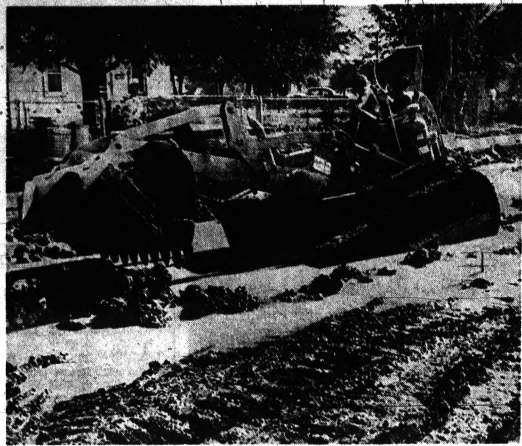
HIS OWN DOING — Ronald Blakeney, a bulldozer operator, sits helplessly on his tractor, bogged down in mud after hitting a water main on a repaving project in Denver. The surrounding area was swamped when the tractor ruptured the main and sank in the mud it created.
