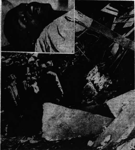
DIG IN RUBBLE — A fireman uses a sledge hammer in an effort to reach men trapped in the rubble of a Chicago building which collapsed Thursday. Three workmen were trapped and 14 injured when walls of the four-story building were being razed.
