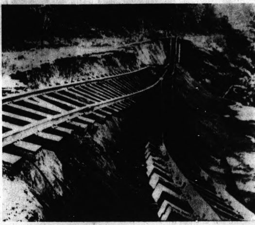
SUNKEN TRACK BED — Railroad tracks near Olympia, Wash., lie twisted after the roadbed dropped as a result of a severe earthquake which shook the Pacific Northwest yesterday. The epicenter of the quake was placed at about 25 miles southwest of Seattle.
