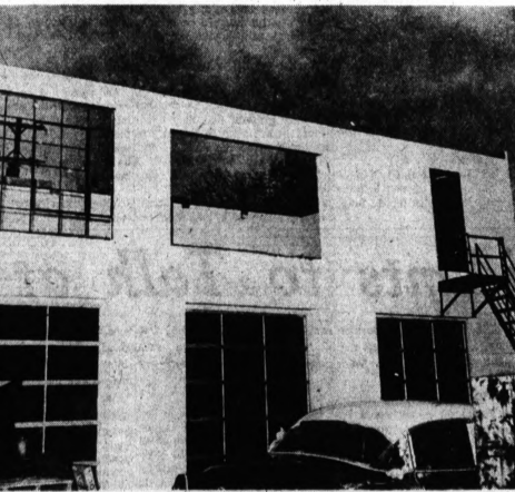
BLEW ITS TOP —Strong winds which whipped through the Pontiac area, throughout the night ripped the roof off this newly constructed garage and showroom at Superior Auto Sales, 550 Oakland Ave. An electric wire shown running over the top of the building also was broken and had to be repaired. The roof was found lying intact next to the auto sales on Blaine Street near Oakland Avenue at about 12:30 a.m. today. Winds reached 32 miles an hour at the Pontiac Municipal Airport last night.
