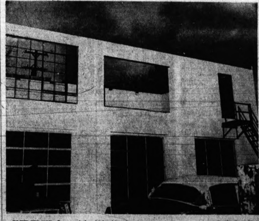
BLEW ITS TOP —Strong winds whipped through the Pontiac area throughout the night ripped the roof off this newly constructed garage and showroom at Superior Auto Sales, 550 Oakland Ave. An electric wire shown running over the top of the building also was broken and had to be repaired. The roof was found lying intact next to the auto sales on Blaine Street near Oakland Avenue at about 12:30 a.m. today. Winds reached 33 miles an hour at the Pontiac Municipal Airport last night.
