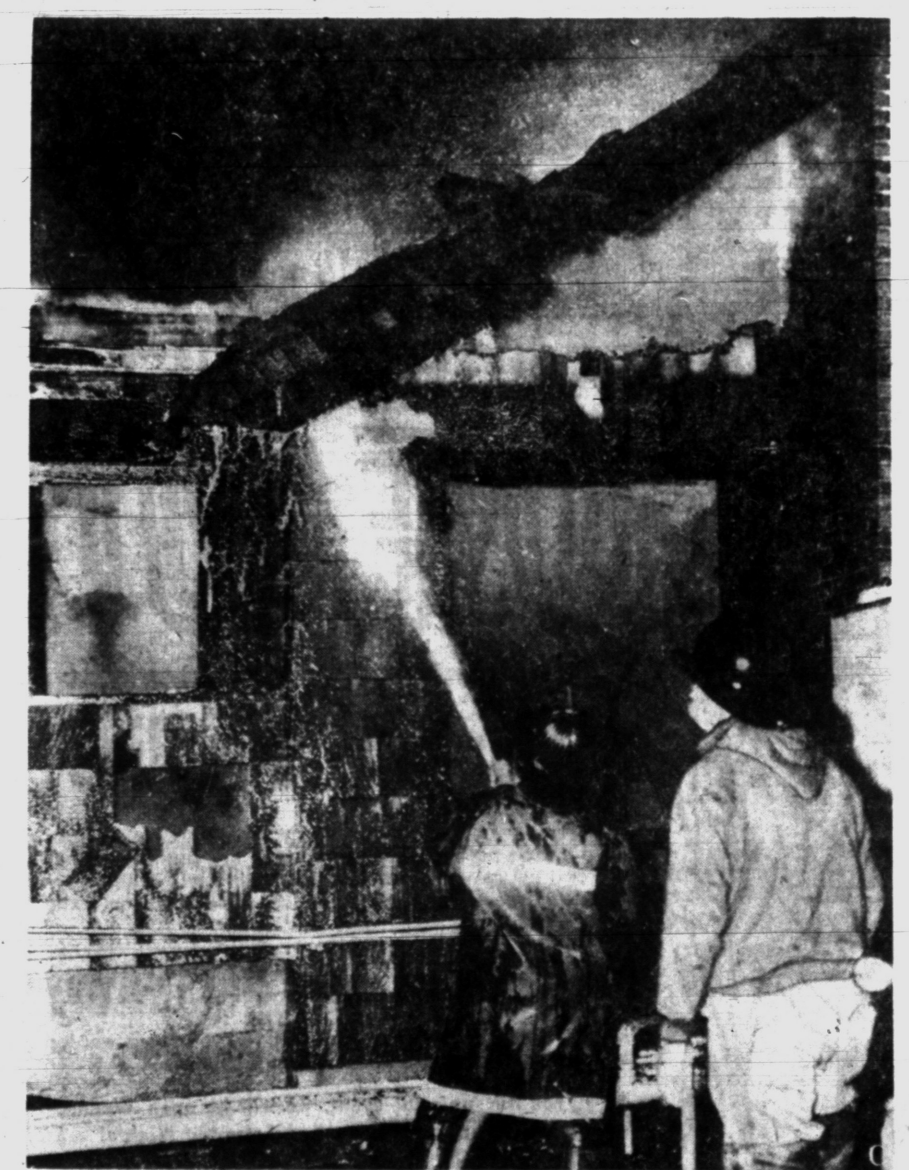
CHARRED REMAINS OF GOLF CLUB HOUSE — Firemen still were at the scene this morning of a $750,000 blaze which destroyed the clubhouse of the Plum Hollow Golf Club in Southfield. Most of the 25,000 square foot spraw-
