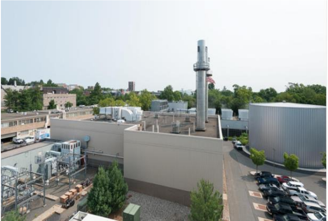
Figure 3.9 Princeton University's CHP plant microgrid [74]
