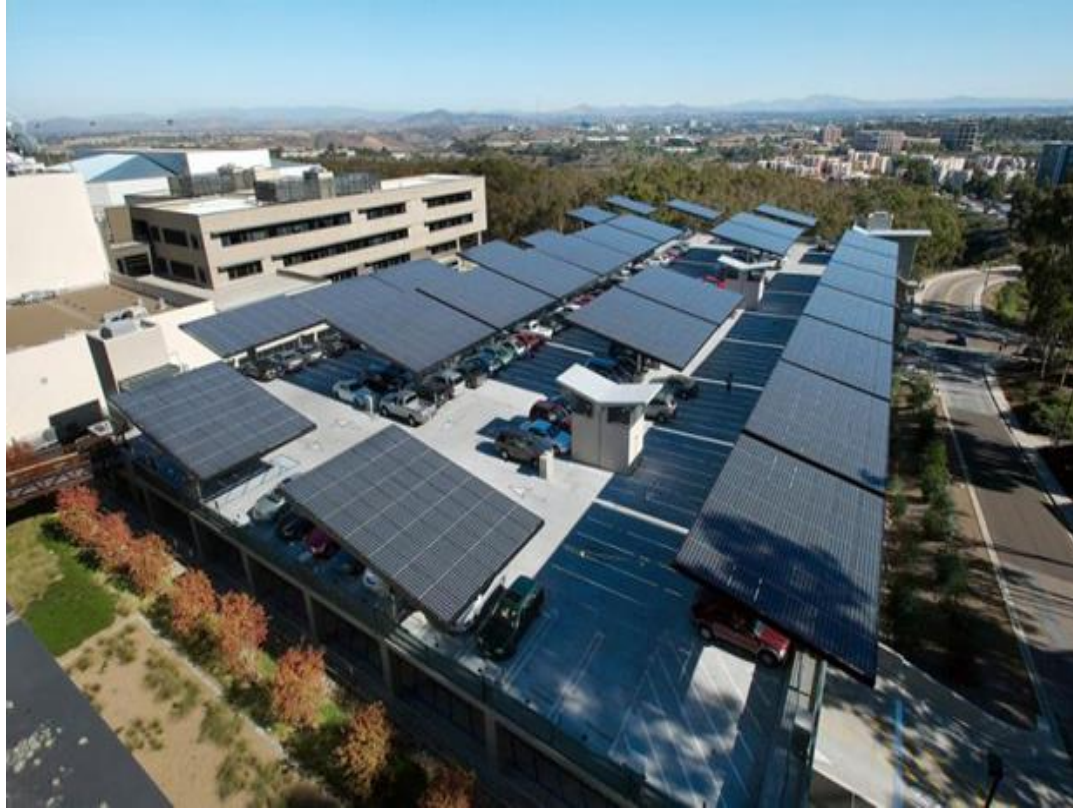
Figure 3.7 Solar panels in the microgrid at UCSD [72]
