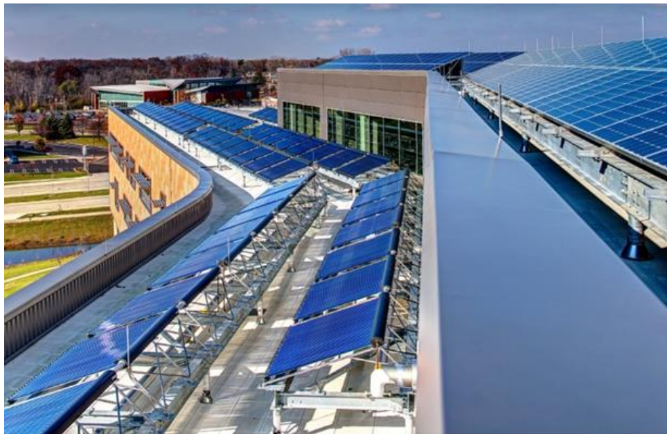
Figure 3.1 Oakland University microgrid [67]
