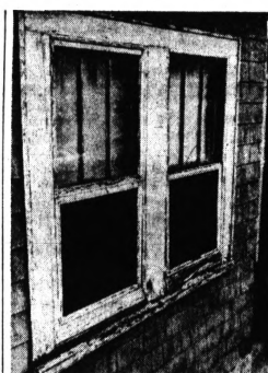
BEFORE: These old unsightly wood windows were rotted, hard to open, let in dirt and air.
