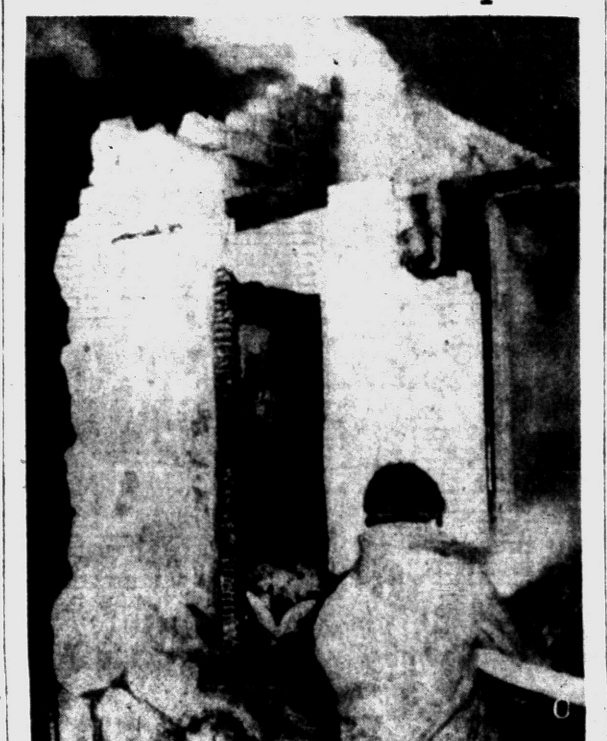
BLAST DAMAGE — A fireman searches the ruins of the Fountain of the World cult building at Chatsworth, Calif. after an explosion which demolition experts said was possibly caused by a bomb early today.
