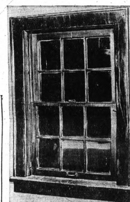
Before Old window is unsightly, hard to wash, rattles, lets in drafts and dirt, has rotted sills and frames.
