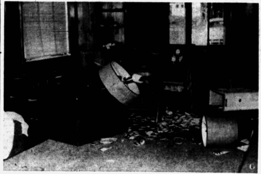
WANTON DESTRUCTION—Above picture shows damage to one of 18 cottages at Woodhull Lake in Waterford Township entered by youthful vandals during owner's absence. This cottage at 4584 Lakeview is owned by Harold Sarko, of 14880 Wyoming St., Detroit.
