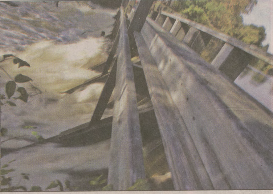
Whittenton Dam is seen Tuesday in Taunton, Mass. An evacuation order was in effect, and schools and highways were closed amid fears of a wall of water up to 6 feet high should the dam fail.
