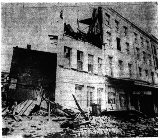
HURRICANE DAMAGE — This building in downtown New Orleans shows the effects of Hurricane Betsy which slammed the Louisiana and Mississippi coasts this morning, causing considerable property damage.
