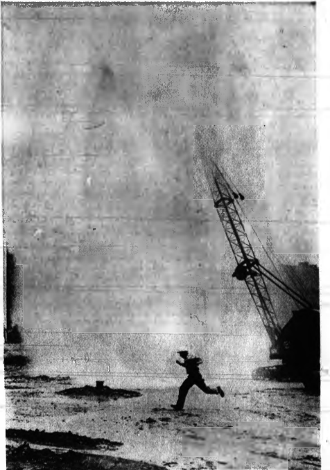
THAT SHE BLOWS — Construction worker's "barrel" riddler heads for cover as water sprays 80 to 70 feet in the air from a crack-d main at a construction site in Omaha, Neb. Bridgford said he was operating a mechanical tamper packing dirt around newly installed sanitary and storm sewer pipes when the machine hit the main. "The next thing I knew I was getting a bath," Bridgford said.
