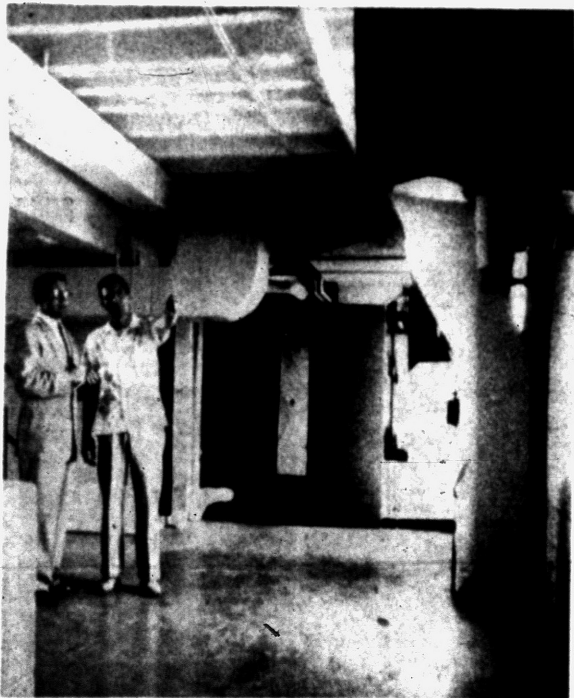
COOLING LOCATION — Ronald Schemel, chief of maintenance at the new City Hall explains operation of equipment in the penthouse atop the million-dollar-plus structure to reporter Arnold Hirsch. Here is located the air conditioning equipment which cools the City Commission chamber and the administrative wing.
