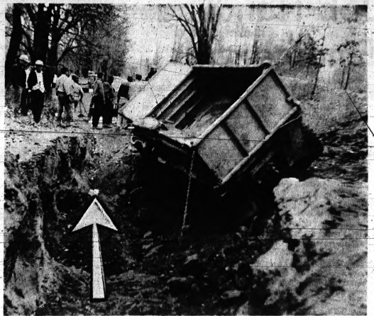
CAVE-IN SITE — Three construction workers were buried (arrow) under an 8-foot avalanche of dirt and a tandem dump truck yesterday in an accident on Squirrel Road south of Square Lake Road, Bloomfield
