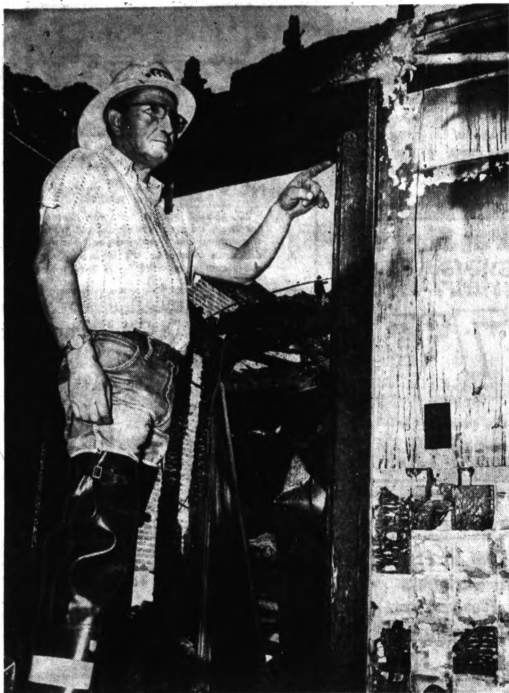
SURVEYS CHARRED RUINS —Lake Orion Fire Chief Jack Caylor points to the blackened door frames and fire-ruined walls in the hollow shell of the Lake Orion Masonic Temple. The two-story building, which houses the
