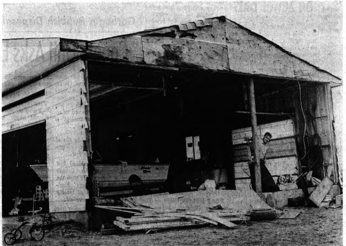
Pontiac Press Photo WOOSH — Kenneth Eubanks of 5136 Mary Sue, Independence Township has quite a blowout yesterday, but it wasn't a party. High winds remodeled his garage, knocking one end of it right out. Here he surveys the damage.
