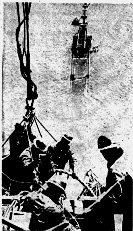
CABLE LAYING MISHAP — Bridgemen are shown laying a mesh-type catwalk on the cables of one of the 552 towers of the new Straits of Mackinac bridge. In a similar operation yesterday a cable of the type in the foreground broke and two men fell to their deaths. Three others scrambled to safety.
