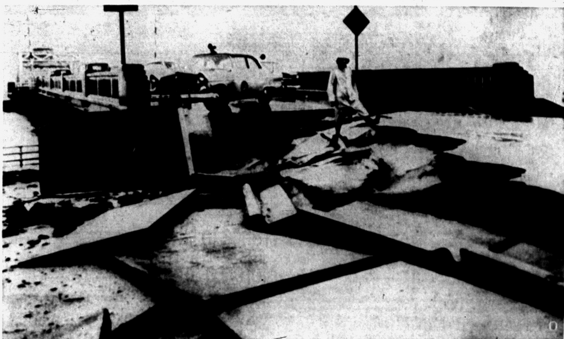
BRIDGE OUT — Hurricane Ione put this bridge out of commission at New Bern, N. C., yesterday as high water washed out the approaches, stranding cars shown on the bridge.
