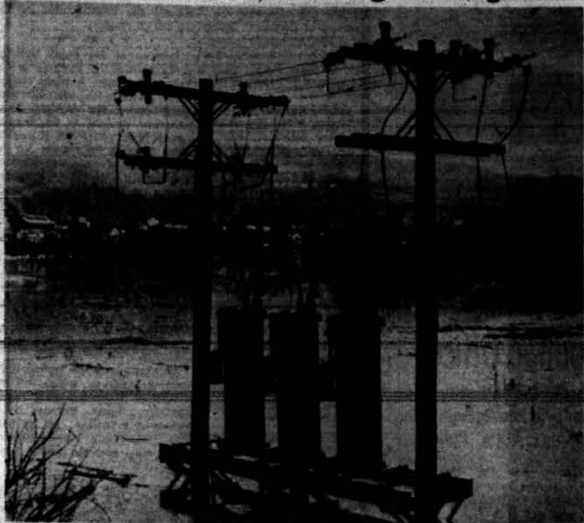
HIGH WATERS —The overflow from the flooding Clinch River in East Tennessee laps dangerously close to a power transformer which serves Hancock County. The flood has marooned several farm families in the region. AP Wirephoto
