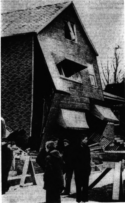
SOMETHING SEAMS WRONG — A tornado which struck Chicago's South Side redesigned this frame home. The front wall took on a bulge at the seams but the building remained pretty
