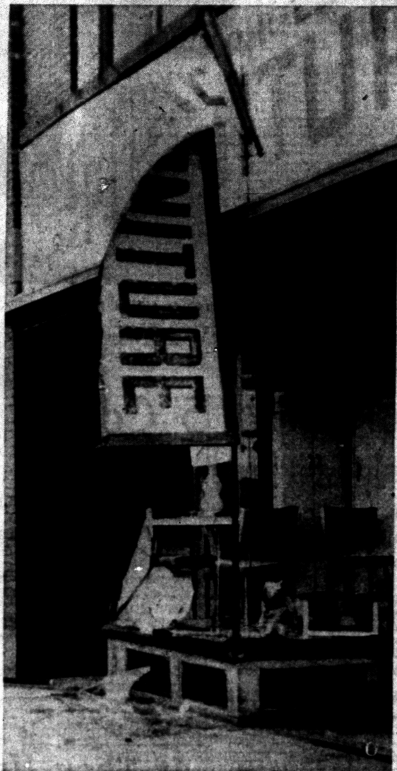
IN STORM'S WAKE — Central Upholstering Co., 105 S. Saginaw St. is left with a broken window and a dangling sign as a result of the driving gale. There was similar damage up and down Saginaw street.
