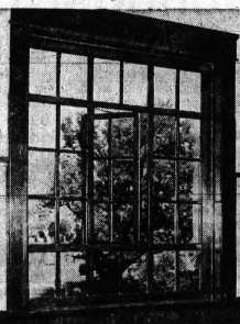
Before This old metal window gave a dismal atmosphere, made maintenance expensive, obstructed light.
