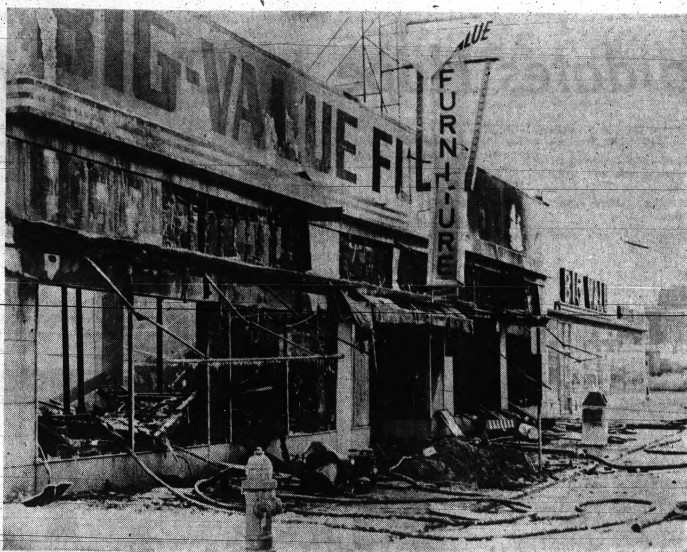
GUTTED —The fire and smoke-blackened store front of Big Value Furniture Discounters, 47-55 S. Saginaw, shows the intensity of the blaze that swept through the building last night. A fire wall kept the blaze from spreading to the adjacent supermarket.
