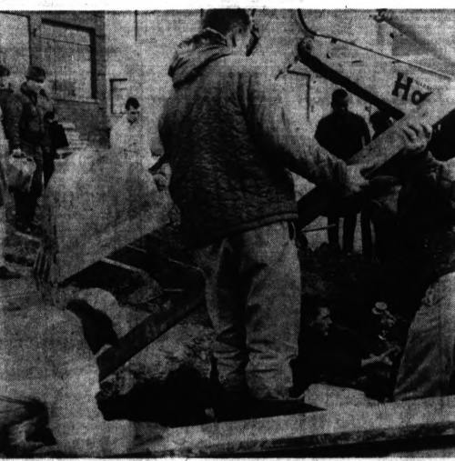
CAVE-IN SCENE — Water Department employees Norvin B. Rasel died yesterday when a ditch he was working in collapsed. Here workers are seeking to free him at the scene at East Boulevard near Perry. He was repairing a water main.
