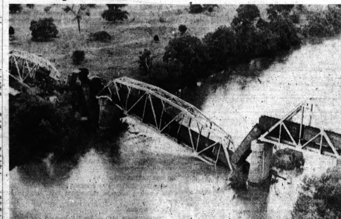
TRAIN WRECKS BRIDGE — This Southern Pacific freight train brought this bridge crashing down into the Colorado River near West Point, Tex., Friday as a load of steel shifted and struck the bridge. Thirty-six cars jumped the track and piled up at one end of the span. The remainder of the 93-car string stopped short of the bridge. No injuries were reported.
