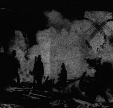
FLAMES AT U.S. EMBASSY—A mid-impressive background of twisted steel arches and smoke, Mexican firemen fight to subside the rampaging fire which destroyed the eastern wing of the U.S. Embassy building under construction in Mexico City. An official estimated damage at $100,000. Cause of the blaze has not been determined. This was to be the largest U.S. Embassy in Latin America.
