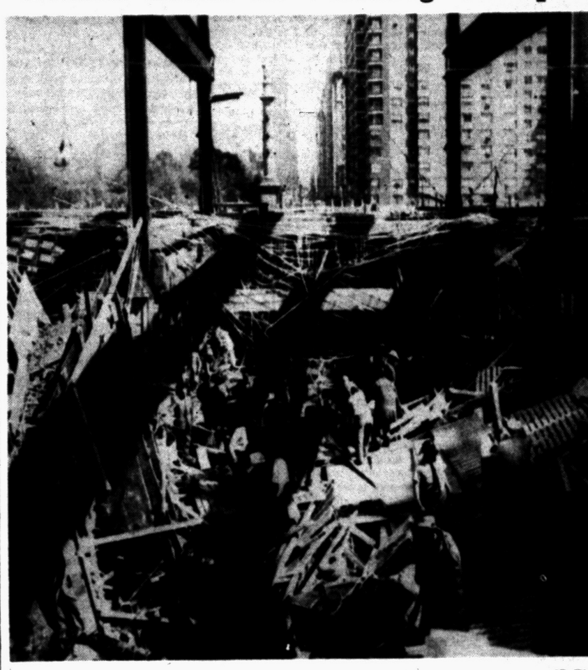
AT NEW YORK COLISEUM — Police, firemen and construction workers hunt through wreckage that crashed 22 feet when center section of exhibit floor of New York Coliseum collapsed during construction yesterday. Of 1,000 at work on the building when the collapse occurred, one is missing and at least 51 injured. About 100 workers were in immediate danger when the accident happened.
