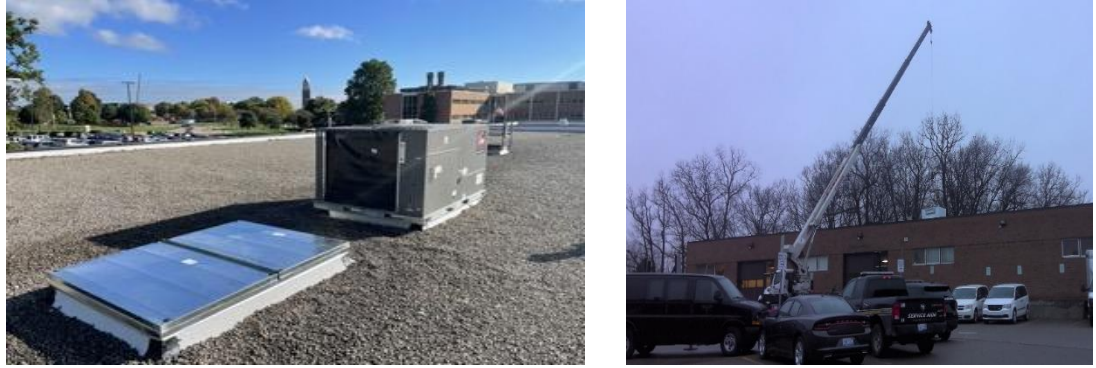
Figure 1.2 The Oakland University Campus Police & Support Services Building with the roof-top unit on the left and the membrane-based energy recovery ventilation system being installed on the right.
