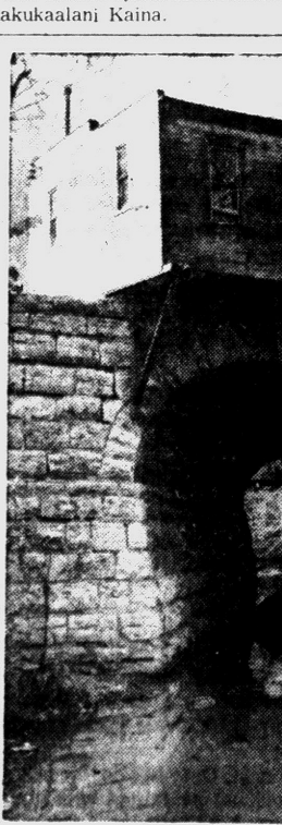
TIPSY LIQUOR STORE — While it appears quite secure from the front, the view from behind this liquor store in Kansas City, Mo., reveals that the rear half of it has a rather unsteady foundation, hanging a number of feet above a creek by the grace of three supports.
