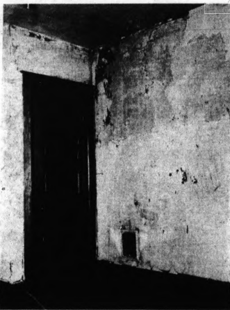
BEDROOM - BEFORE — The photo at right, taken a year ago, shows the condition of a bedroom in a home at 133 Judson St. If you think it was beyond help, see the picture below.
