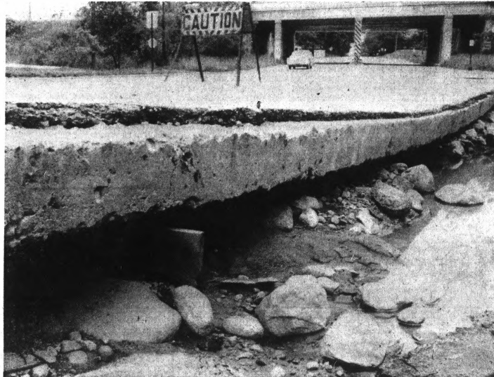
Damaged Long Lake Road, One Mile East Of Woodward
