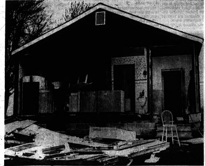
Demon Winds Peeled Off Back Wall Of Lunsford Home On Joslyn
