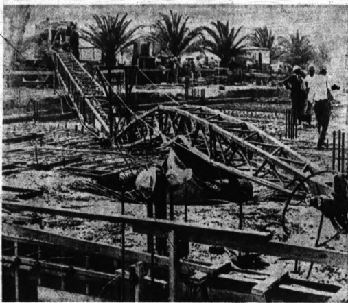
FIVE DIED HERE — A bucket loaded with two tons of cement (half hidden in center) came crashing down killing five construction workers yesterday when a cable on this crane snapped. They were working on a construction project at
