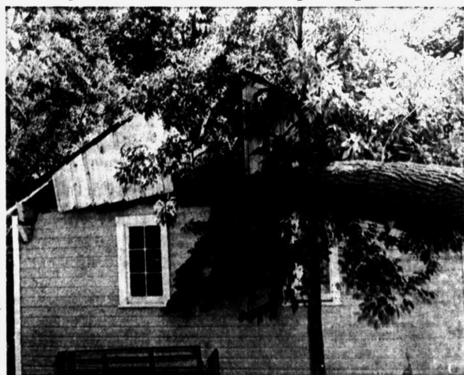
WIND DAMAGE — Winds clocked at 65 miles an hour in Saturday's savage thunderstorm toppled this big elm tree onto the garage at the home of Joseph R. McCarthy at 300 Draper Ave. McCarthy's car, parked partly inside the garage, was undamaged.
