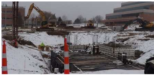
The School of Engineering and Computer Science's new Engineering Center is coming along nicely since breaking ground. Building crews are forming the foundation in the snow and cold
