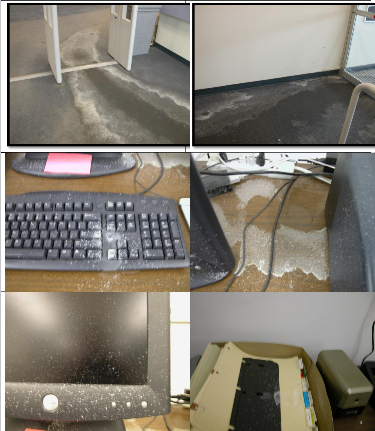
Photos documenting the problem and damage:
