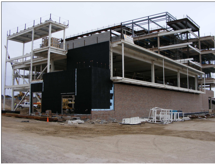
The School of Engineering and Computer Science's new Engineering Center continues to come along nicely. This photo was taken recently from the Science and Engineering Building.
